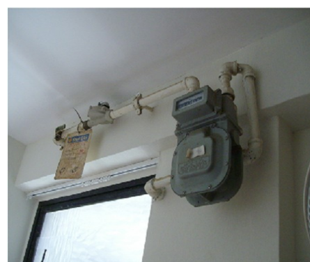
LPG meter inside a domestic apartment
