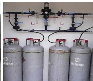
Bank of 45kg cylinders supplying a metered facility
