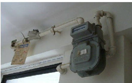
Metered LPG supply from cylinders
