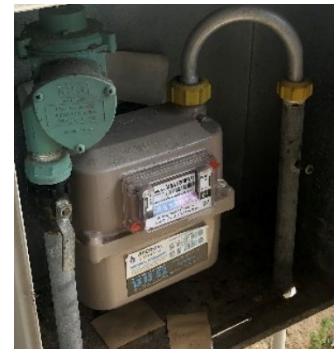
Meter located outside
